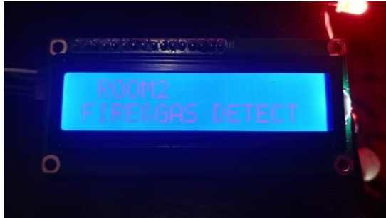
Gambar 16: Fire and Gas detect
